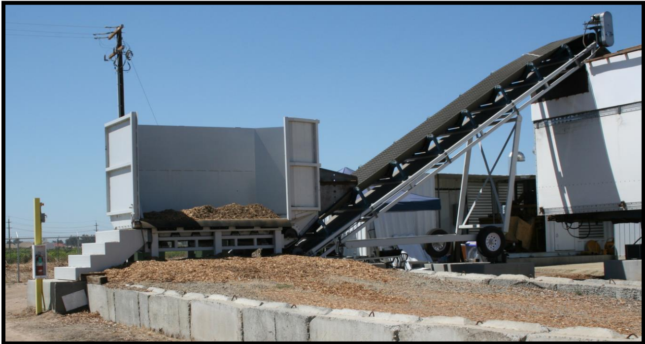
Figure 17. Phoenix Energy Feedstock Receiving System
