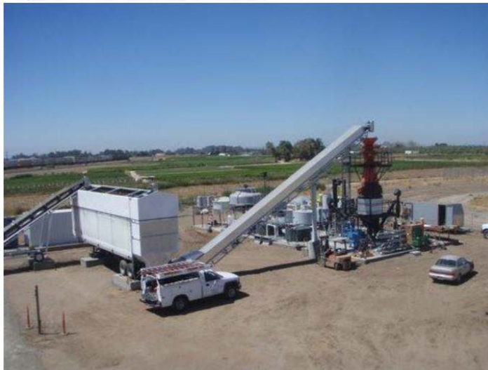
Figure 3 – A P500 installation in California
