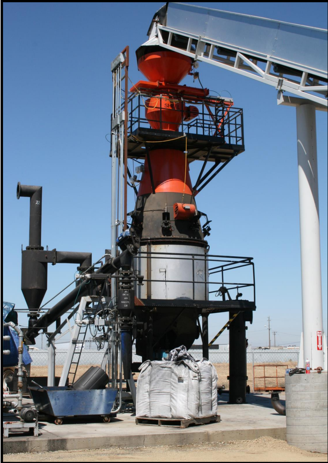
Figure 18. Phoenix Energy Gasification Equipment
