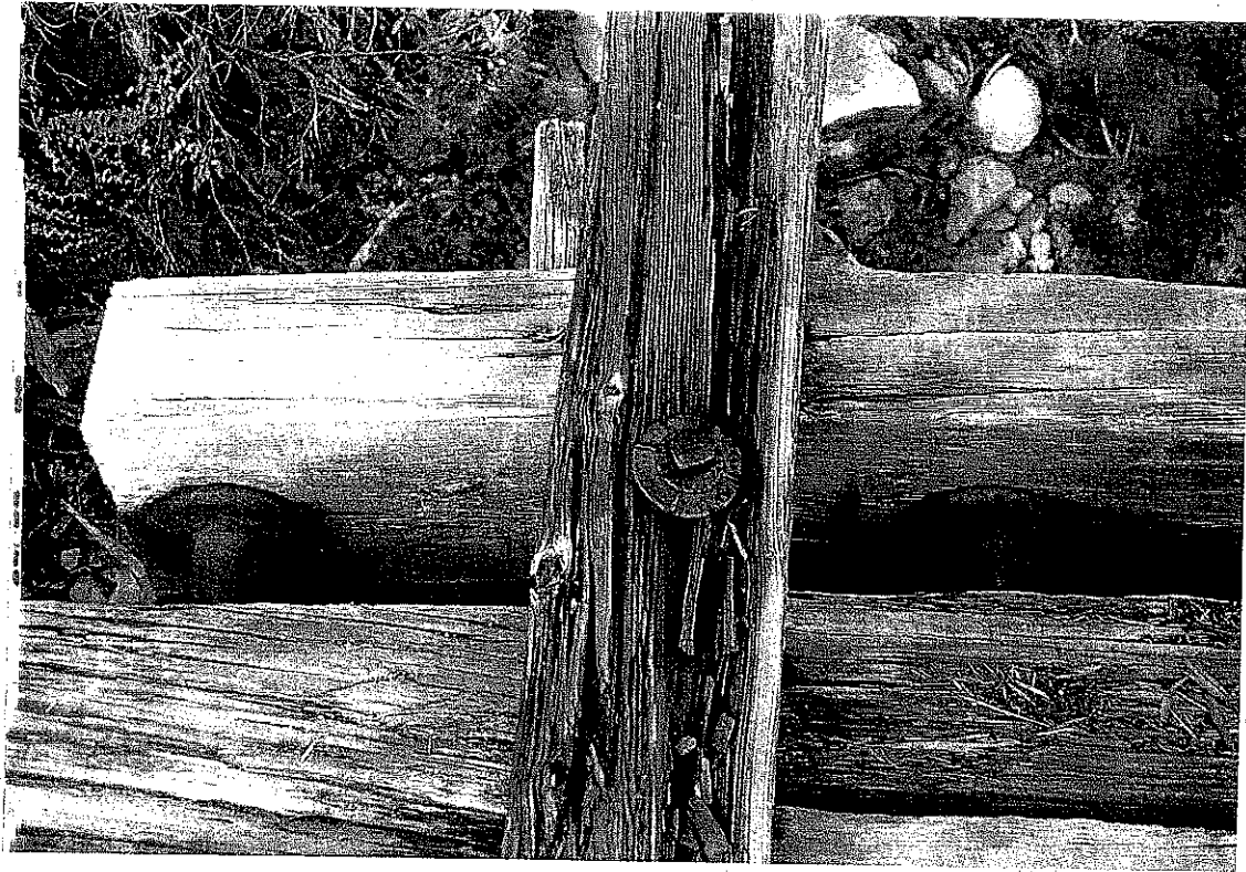
Dry rot, cast iron hardware, and bolted connection
